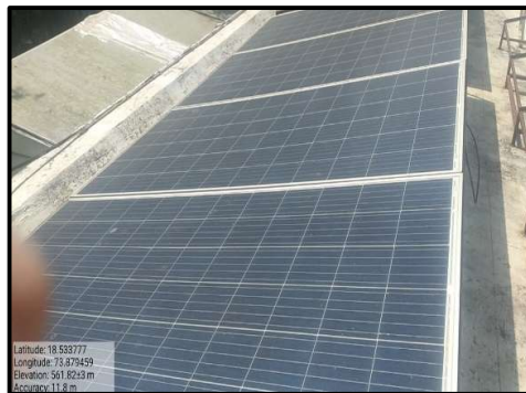
Photograph of Roof Top Solar PV Plant:
